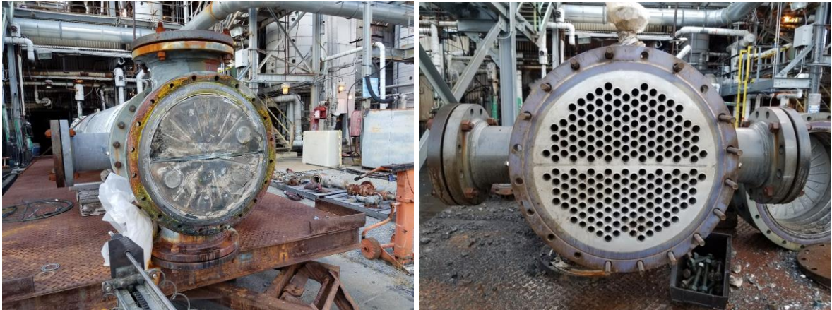
Figure 3. Exchanger prior to cleaning (left) and exchanger channel head removed, completely cleaned with NitroLance (right)
