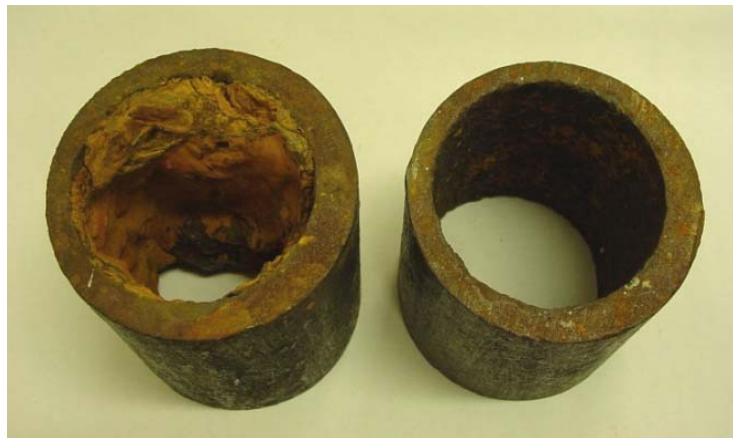
Fig. 12. Exemplary effectiveness of water pipe cleaning (approx. 60 years old cast iron pipeline, nominal inside diameter 100 mm)
