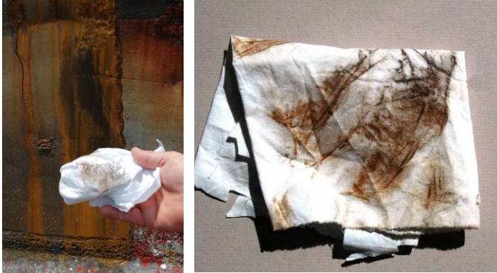
Figure 8 Heavy Flash Rust. Black rust under the light brown rust. The surface is obscured. A layer of RUST SCALE has not formed
