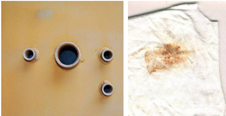
Figure 7 Moderate Flash Rust. Hand Wipe. Note: Tape test on upper left. There is no black rust under the lighter brown rust.
