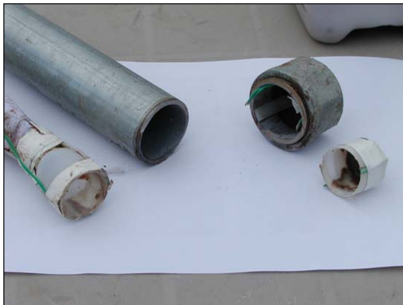
Figure 6. Cut pipe with evidence
