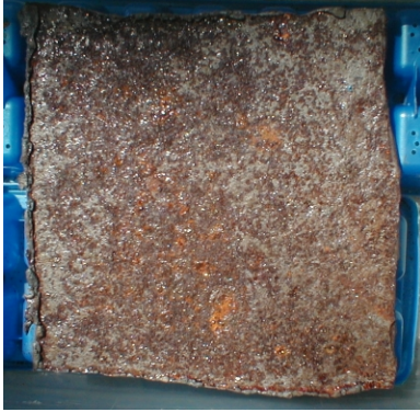
Figure 5 Marine Steel Pressured Washed, Then Abrasive Blasted Exposed to Humidity 6 years later
