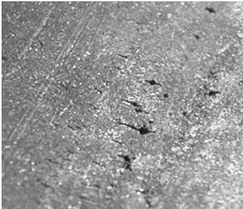
Detail of Corrosion Pits in Stainless Steel Tube Figure 2.
