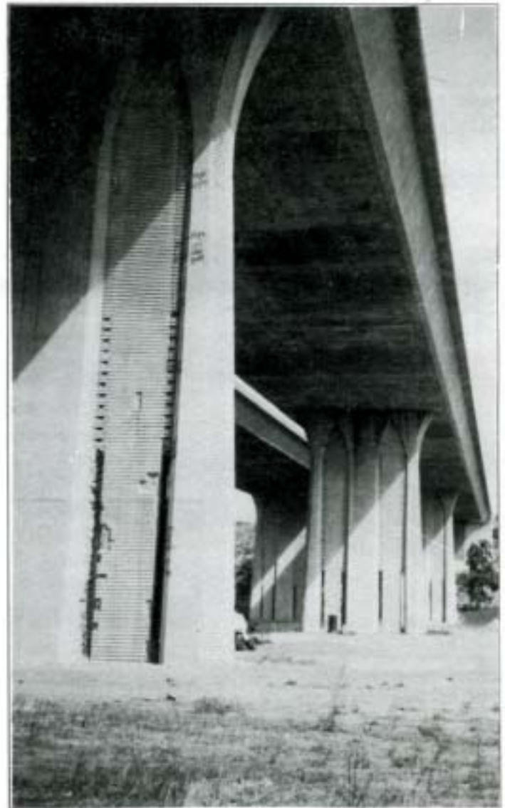
This photo shows four of the pillars in which slots were cut.
