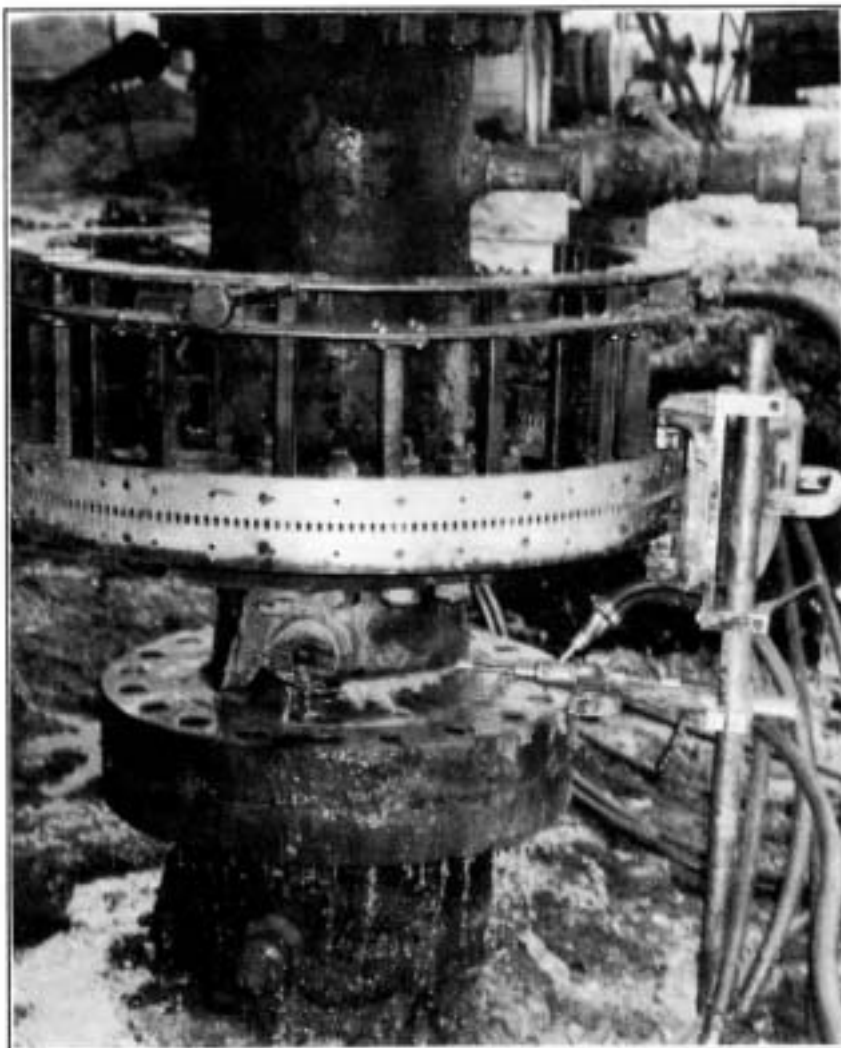
Abrasive jet cutting through orifice well head casing on an extinguished well in Kuwait.
