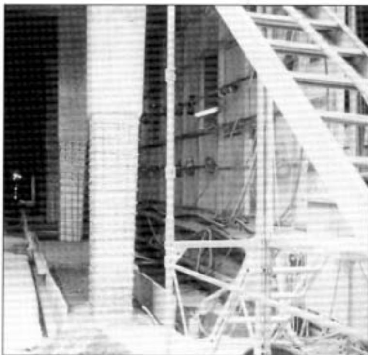
Gallery-pillars after the reinforcement is exposed by mechanized waterjetting. Photograph courtesy of WOMA Corporation.
